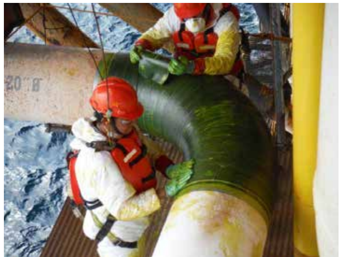
Technicians apply Thermo-Wrap™CF, a custom engineered high strength carbon fiber composite, on a 20" OD elbow of an offshore oil platform located in Brazil.
