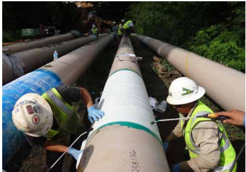
Scar-Guard™ application on multiple welded field joints of a 24" OD natural gas pipeline located in the USA.
